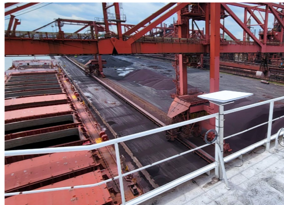
Starlink Maritime installed on the Algoma Sault
